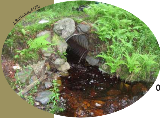
Culvert found in Kejimikujik with insufficient water for fish passage
